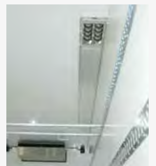
Roof Duct System
